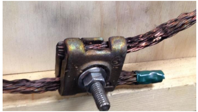
Figure 3. Source conductor movement on PP3C
