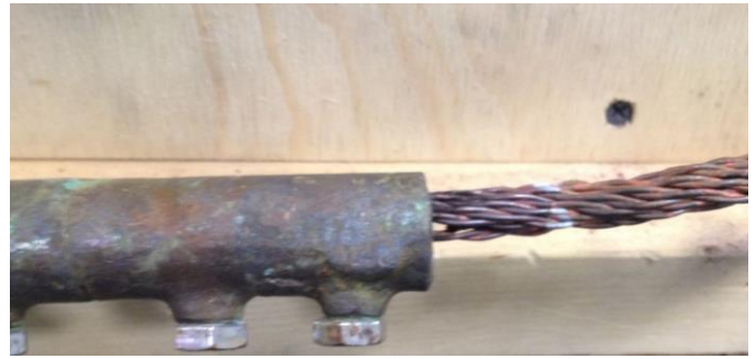
Figure 2. Movement of conductor from Connector AS1C. Conductor movement is distance from connector body to white stripe on conductor.
