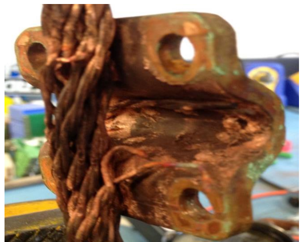
Figure 4. AT1C showing broken strands with missing source conductor.
