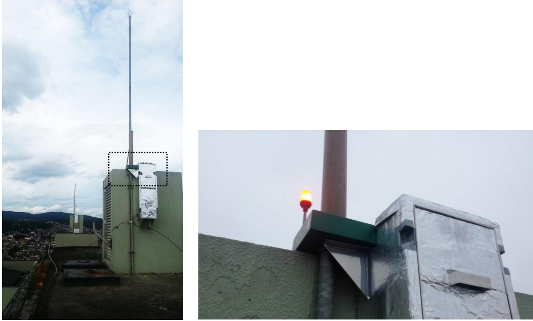
Figure 5. Current sensor installed on the lightning rods (left) and detail of the installation (right).
