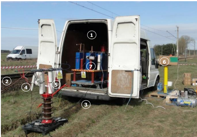
Figure 4. Surge generator post:
